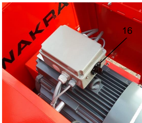
Figure of the main switch
